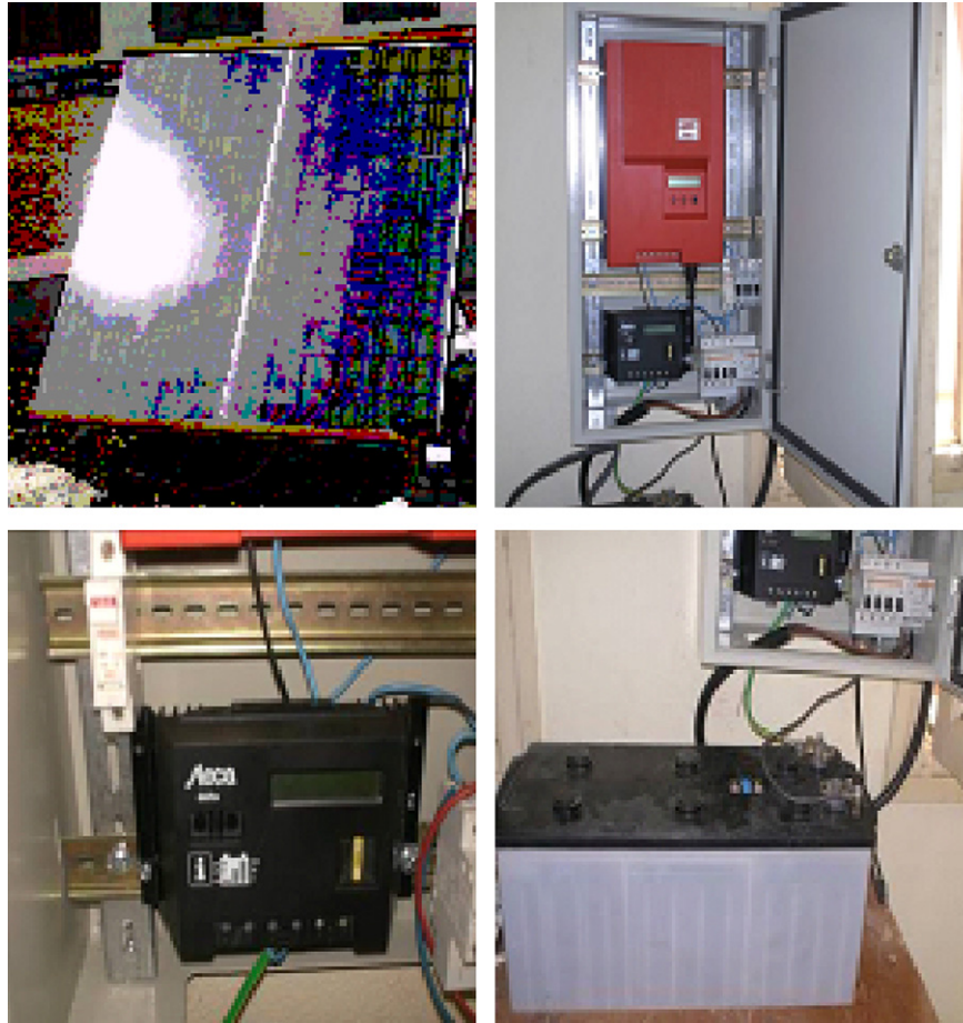
Fig. 3. PV array structure, controller, inverter and battery.
